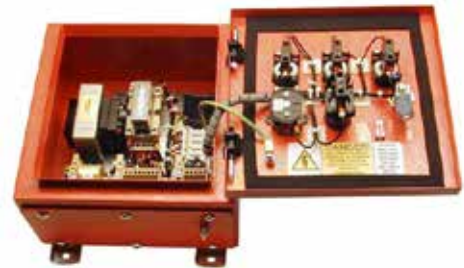
CS1 Control Station Interior
