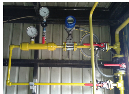
Vortex flowmeter mounted in a bypass line
